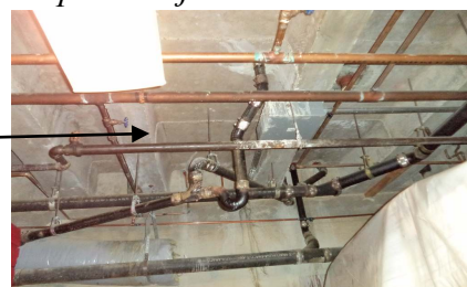
Some of the Deteriorated Waste Lines and Pipes
