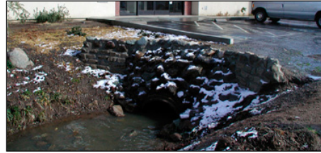
A seasonal creek at the Tuolumne Branch Library is adjacent to the entrance. It lacks a protective barrier.
