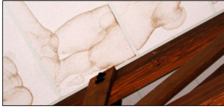
Water damage to ceiling tiles at the main library due to a leaky roof.
