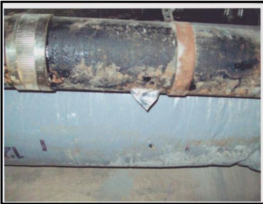
Figure TCJ-1. Evidence of pipes and plumbing in severe disrepair. These conditions are commonplace at the current Tuolumne County Jail facility.
