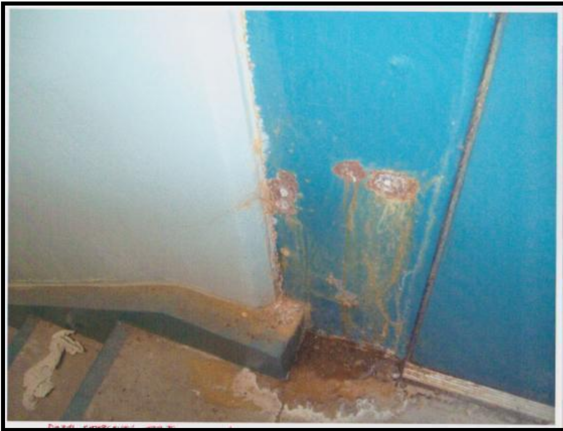
Figure TCJ-2. Evidence of water damage to walls. These conditions are commonplace at the current Tuolumne County Jail facility.
